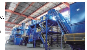
ASR Recycling Facility
