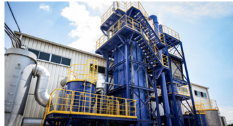
Environmental facilities at the Fujinomiya plant
