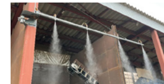
In-plant measures to control dust
