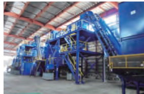
ASR Recycling Facility
