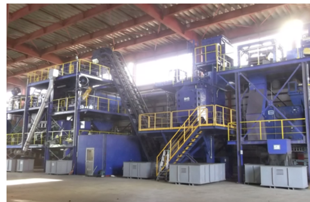
ASR recycling plant
