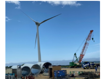
Wind power generation facility
